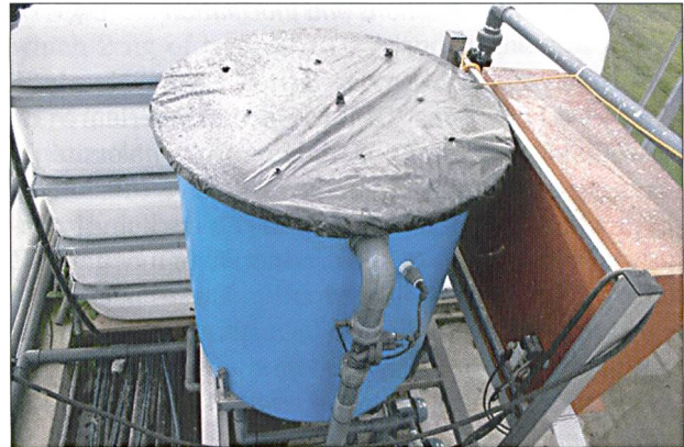
Fig.2: A. Slow sand filter (SSF).
