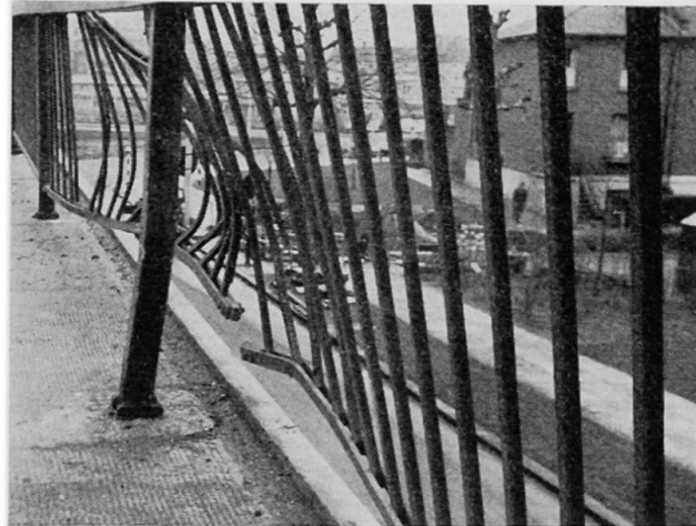
Fig. 10. Damage to bridge parapet railing after impact from sports car.
