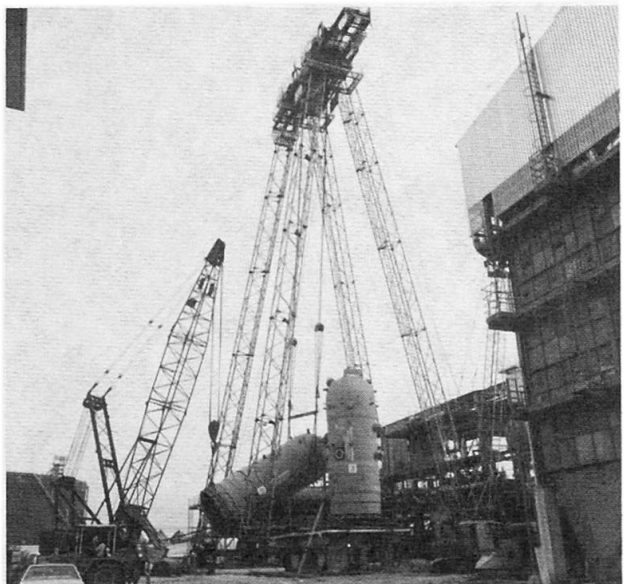
Fig. 4 Lifting frame during the erection of 2 reactors with a weight of 250 t each, in Malaysia
