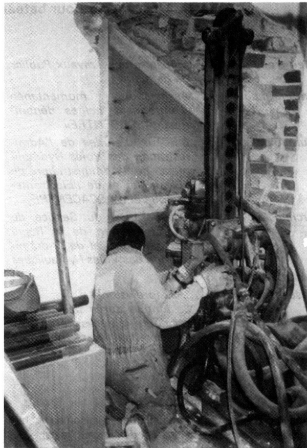
Fig. 2 Through excavations in the supportive brick walls holes were sunk vertically through the basement walls.
