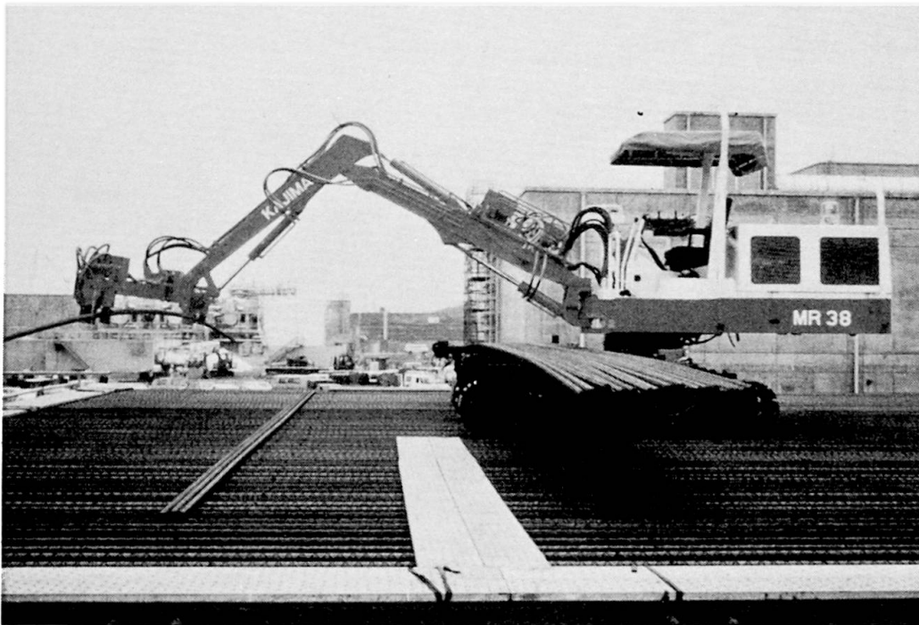
Photo 1 Heavy bar assembling robot
