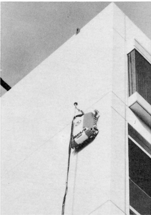
Photo 21 Wall inspection robot
