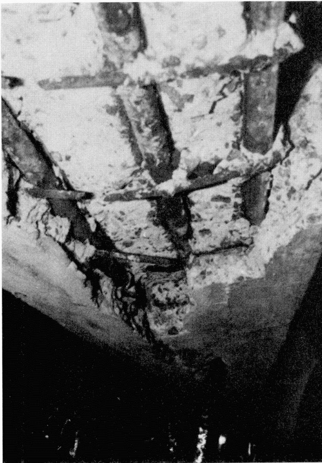
Fig. 4 Corrosion of concrete with expansion
