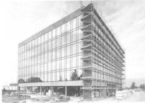
Fig 6 Building "Tour Balexert" at Geneva. All windows and curtain wall in "High Insulation Technology". No heating, only ventilation at 20-22°C.
