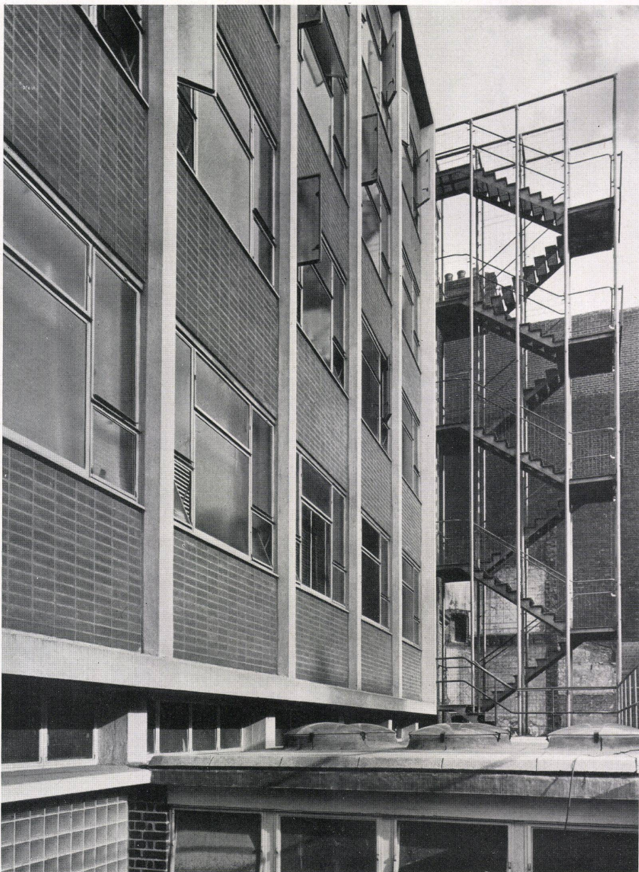
Detail of the facade showing skylights over the yard structure and new stairs.
