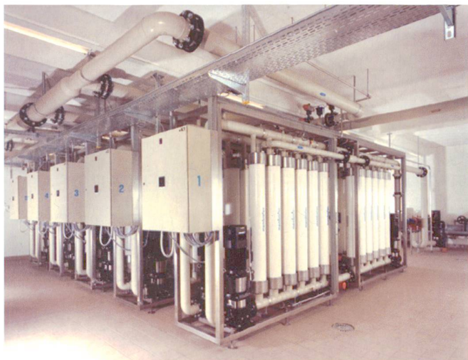
UF-Anlage Lens/Crans-Montana, 450 m 3 /h.
