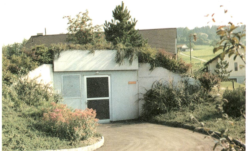
Hangeinbau-Trafostation EW Gossau
