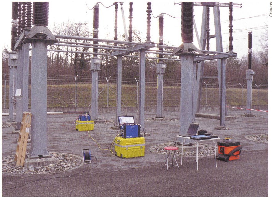
Figure 3 Infrastructure de mesure.
