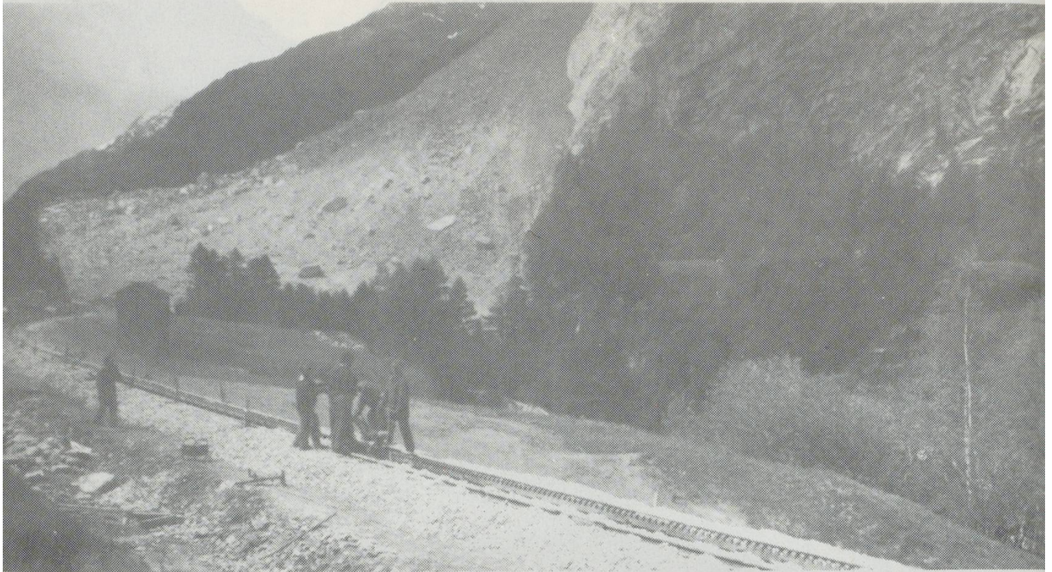
Above: Work progressing on the realignment of the BVZ above Herbruggen, 8 June 1991.
