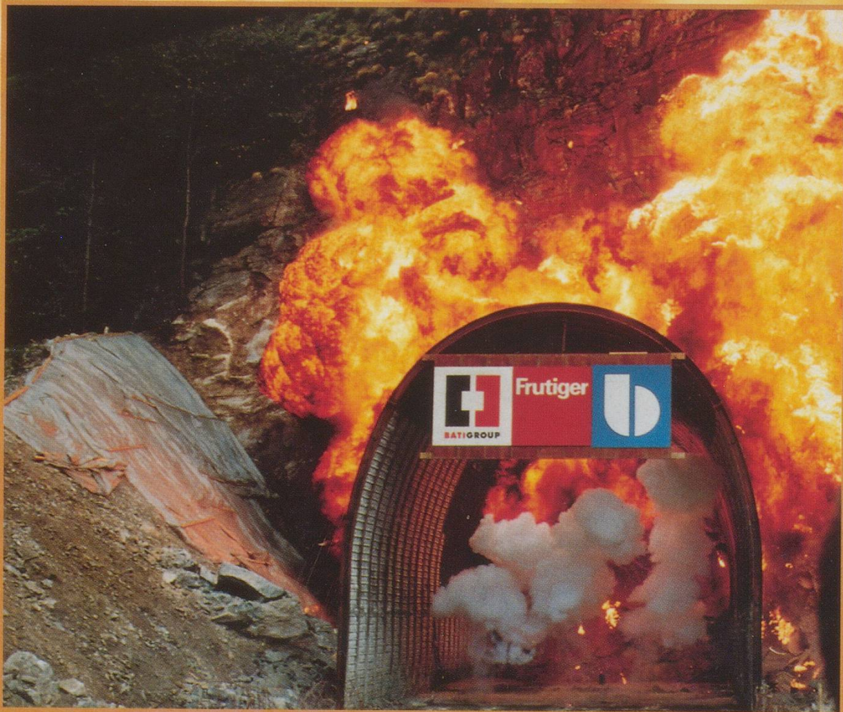
Definitely a photo needing colour for impact. George Hoekstra was bang on the mark with this one. "The Big Bang", The first blast on the Southern end of the new Gotthard Base Tunnel in Bodio on the 10th July 2000
