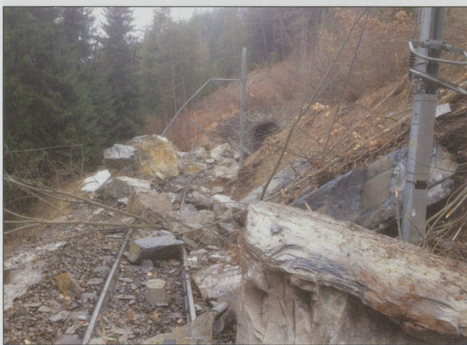
Chur - Arosa line blockage.
