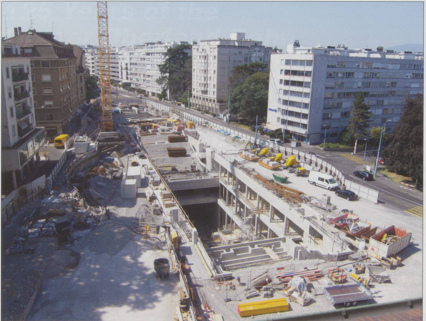
Construction of the future Champel-Hôpital stop. The opposition to the CEVA project was the fiercest here as the station is being built on the site of a neighbourhood park. (19.9.2015)
