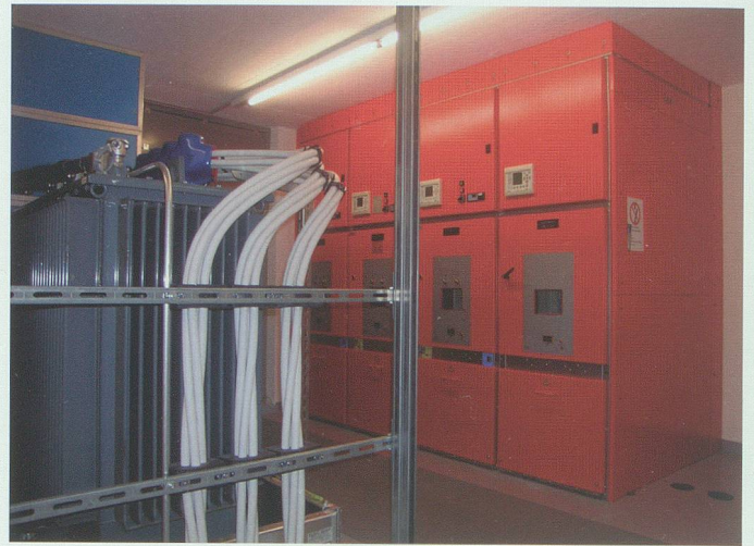
Blick in die Trafostation Witi in Buchs. Foto EWB
